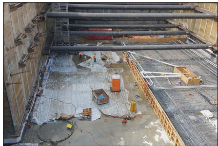
Figure 11. Construction of 1st/Central Station invert
