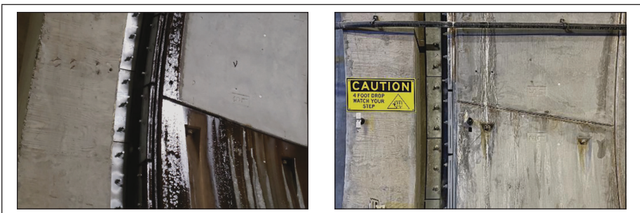
Figure 25. Water leaks at 2nd/Hope tunnel interfaces before and after leak repair
