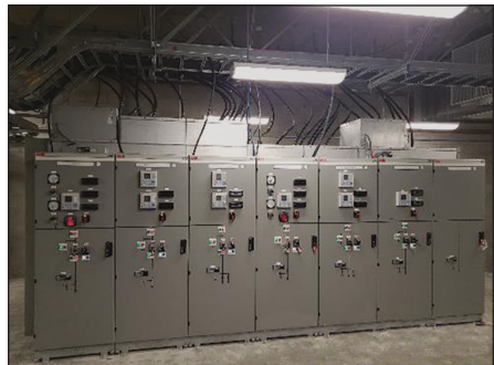
Figure 24. Traction power substations room
