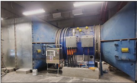
Figure 21. Emergency ventilation fan installation
