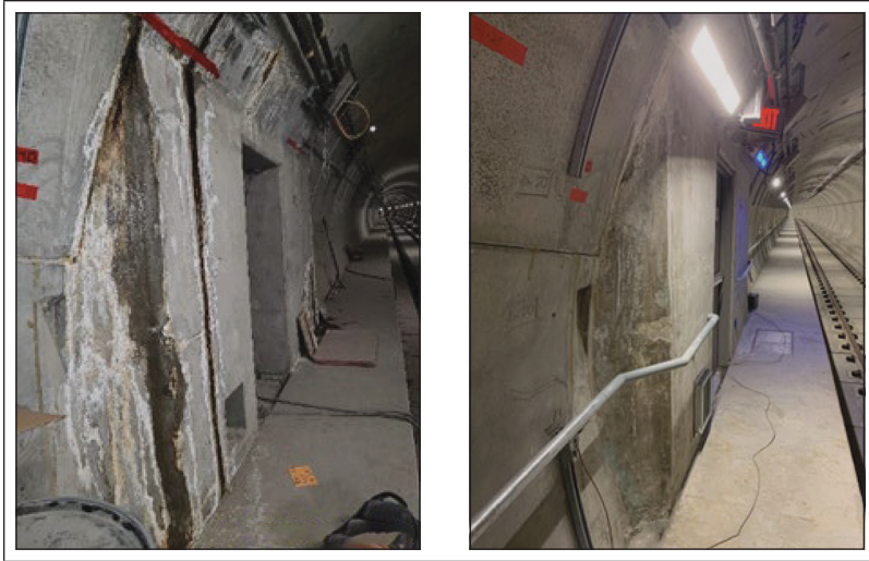
Figure 26. Cross passage CP3 water leaks before and after leak repairs
