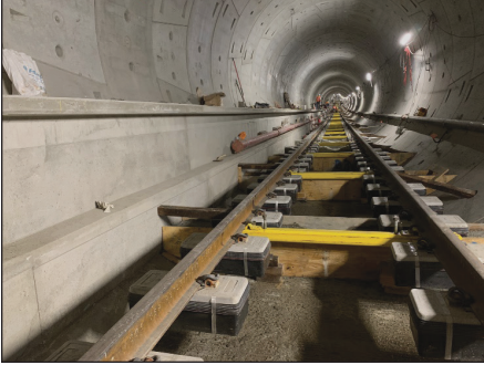
Figure 19. LVT rail system with strong back support
